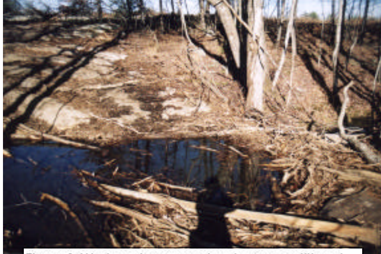
Figure 2. Western stream crossing. Large quantities of logging debris has been left in this stream. Some debris had collected at right of photo forming a dam.
