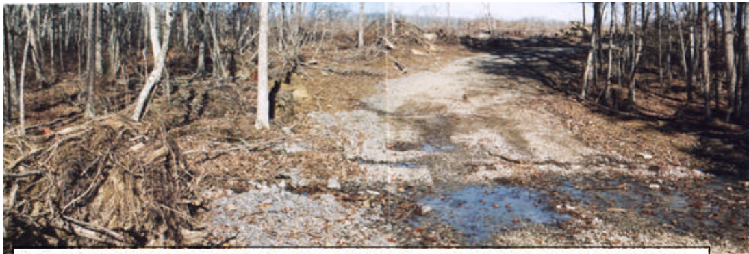
Figure 1. Eastern Stream Crossing. Root ball and debris at left is damming the stream which is forced to seep through gravel placed in the stream bed. The gravel has raised the level of the stream bed and causes the water to disperse
