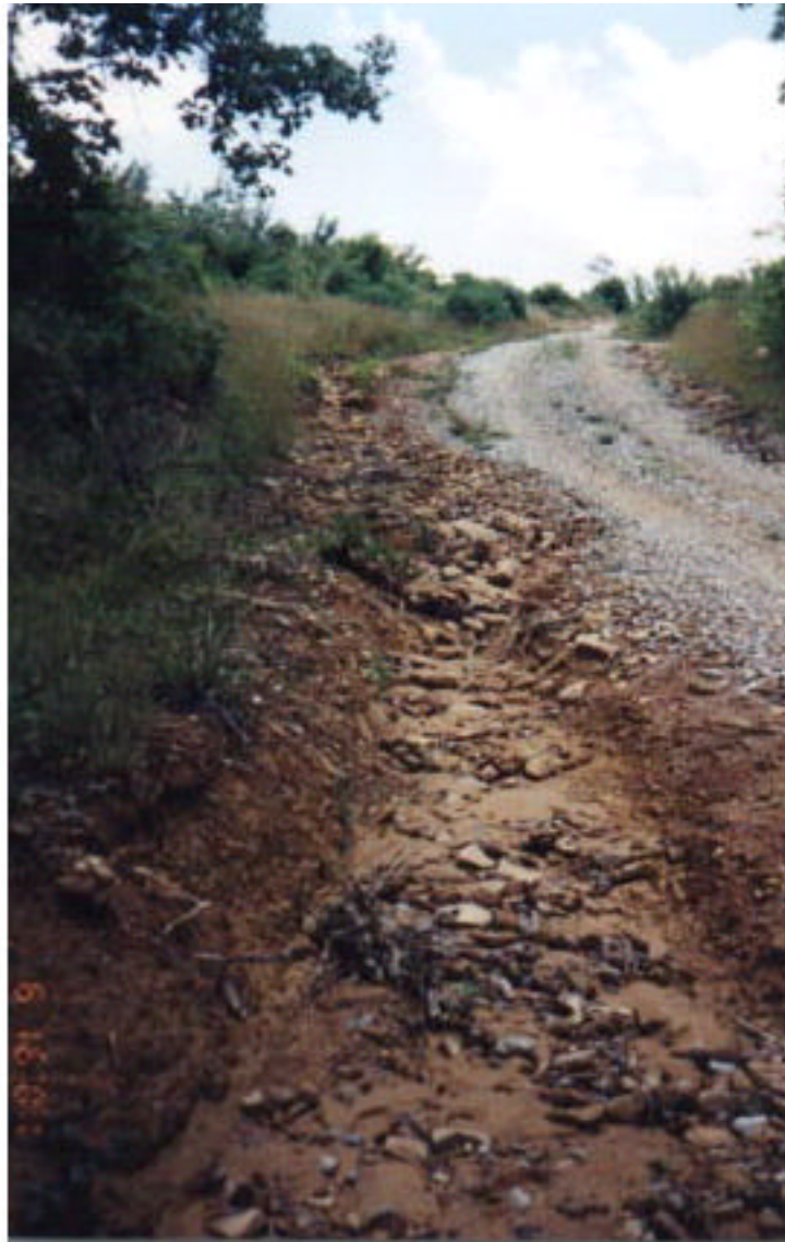
Figure 2. Erosion Channel beside road above the stream crossing. This channel is delivering silt directly to the stream.
